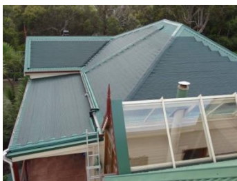
Figure 7: Colorbond™ metal roof with Heritage green Venetian solar collector, Note the Multiple Roof Surfaces.
