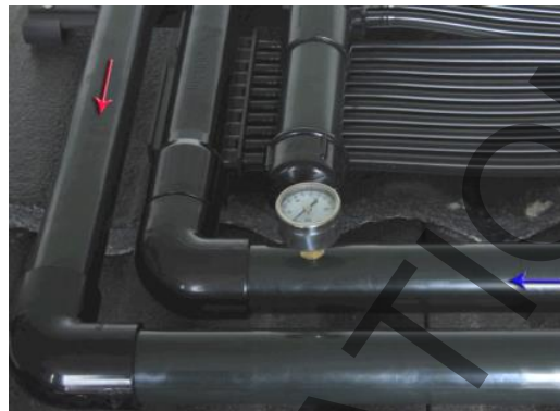
Figure 82: TufGauge™ installed in the Supply Pipe
