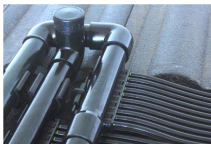
Figure 12: Manifold And Flow Balance Pipe Assembly. Note the VacRel VRV on top of the TufMan Supply Manifold.
