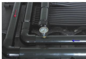
Figure 62: Plumbing at the Bottom of the Manifold System
