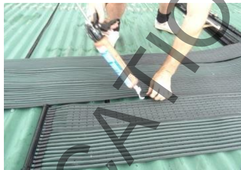
Figure 74: Applying a generous amount of TREMSil® silicone between the roofs surface and the underside of the collector
