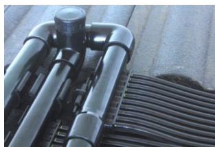
Figure 61: Plumbing at the top of the Manifold System
